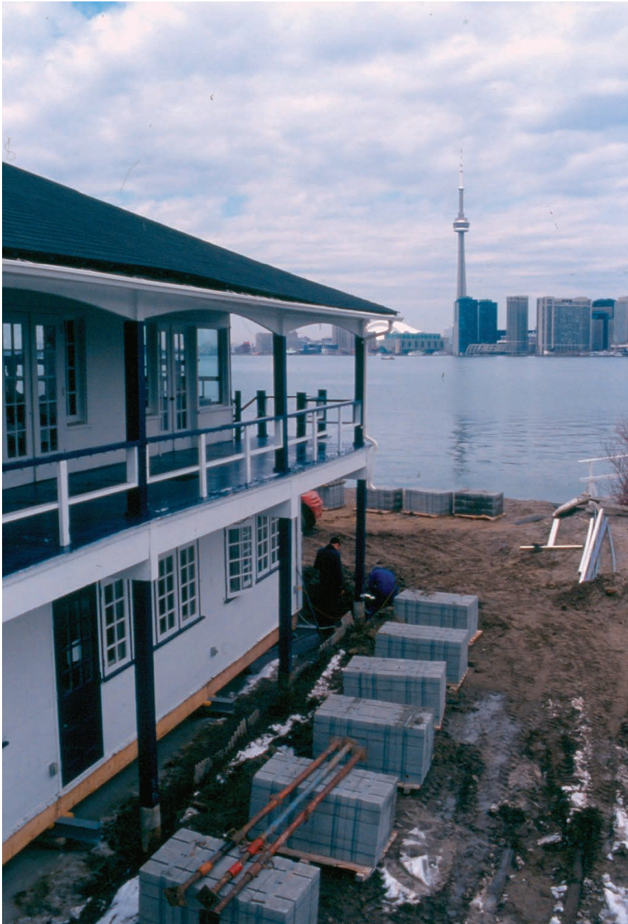
Queen City Yacht Club members prepare for repairing the clubhouse foundations in 1995. Photo Ron Mazza
